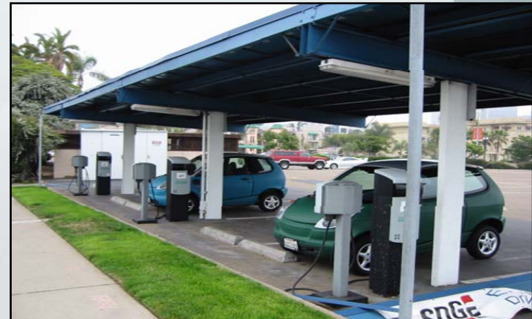
10 kW EV Charging Station
